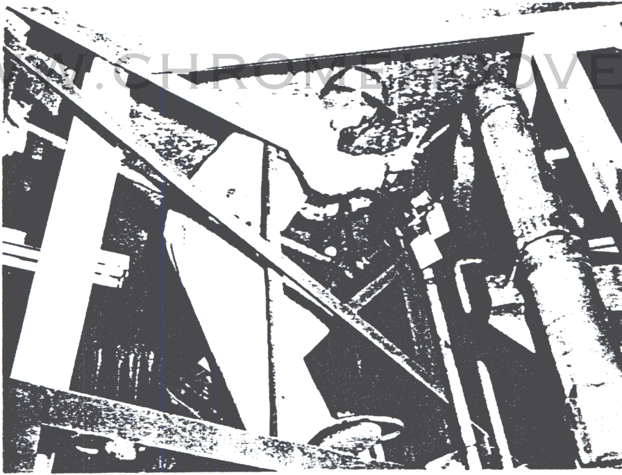
PLS installation in the propellant terminal showing support system for vent lines on upper floor.
