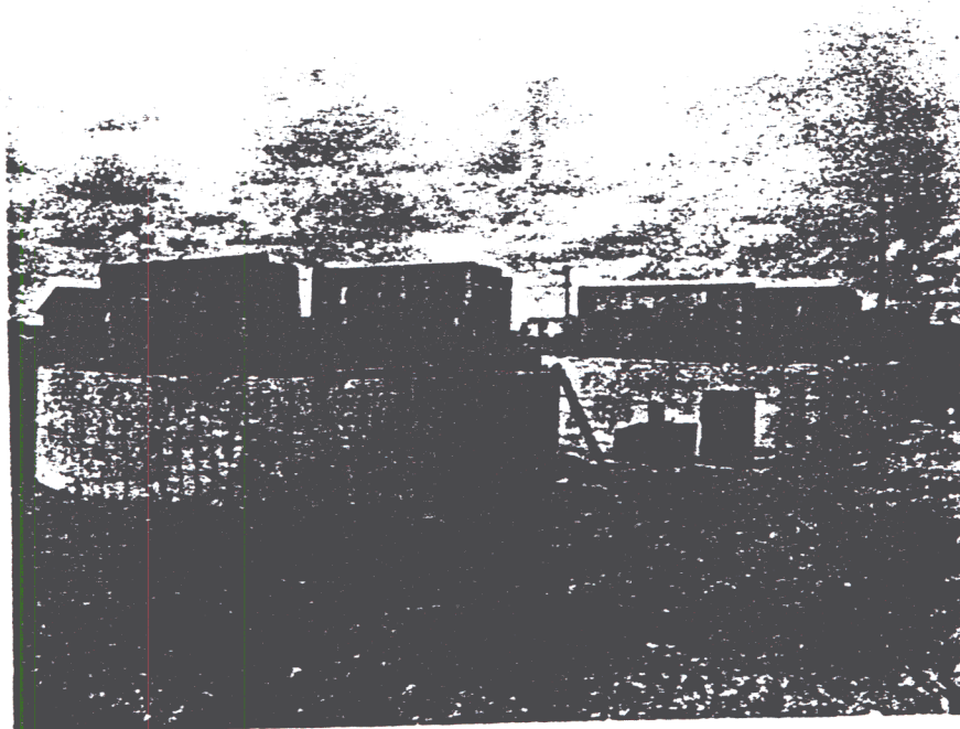
Antenna silo doors installed and tied open. Finish grade will be top of concrete for silo.
