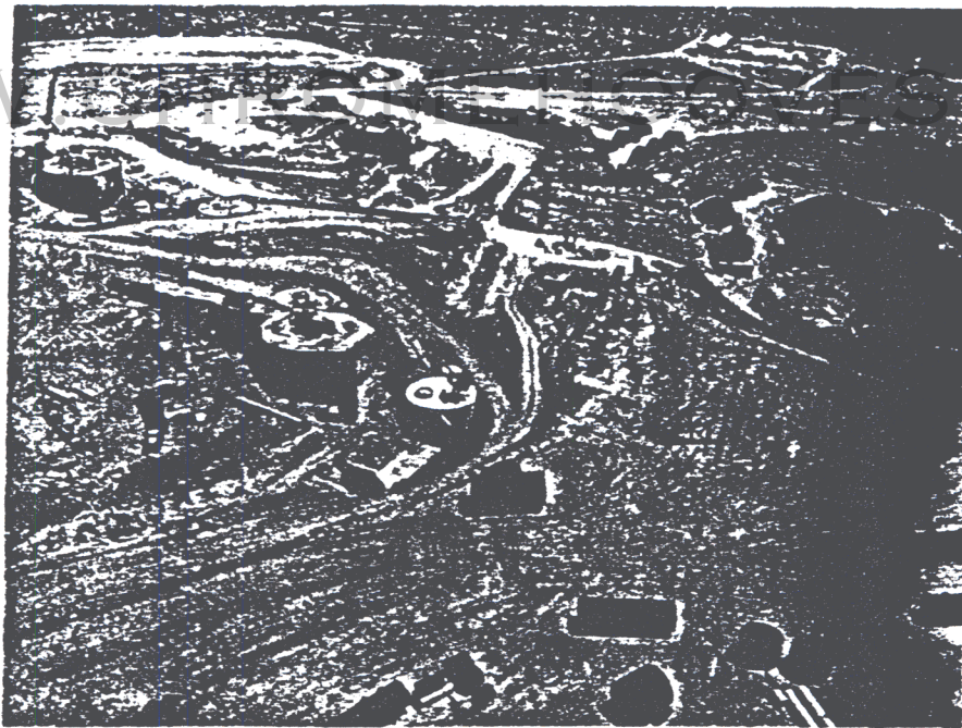
Typical aerial view showing progress to August 1960 showing much of tunnel in place and backfilled. Remaining prefab tunnel sections and junctions in foreground are awaiting placement.
