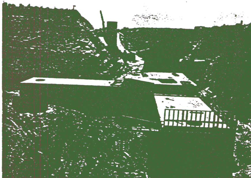
Blast Lock No. 1 placed. Note forming for Blast Lock No. 2 in background.
