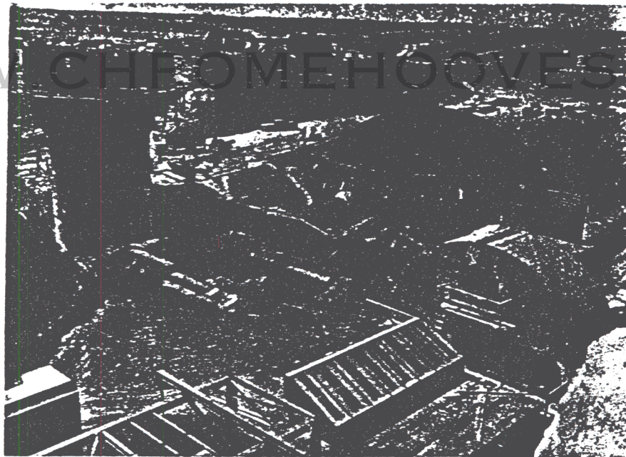
Portal Silo under construction prior to backfill. Note tunnels and fuel tanks in place.
